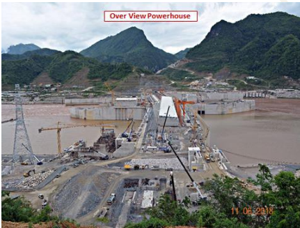
Over View Powerhouse
